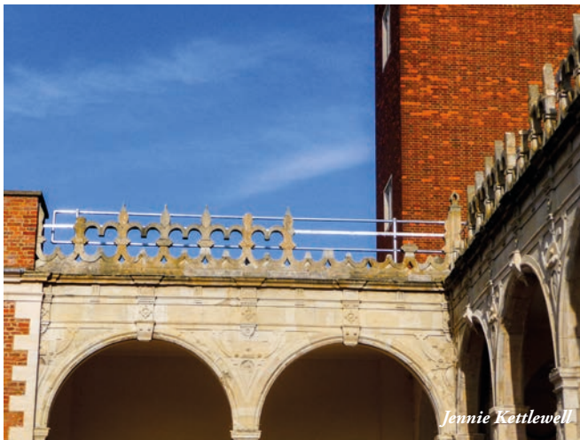
Broken fleur-de-lys balustrades
